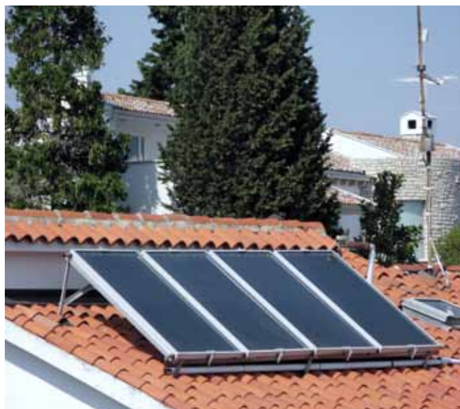
Illustration 4. Solar water heaters on a roof
